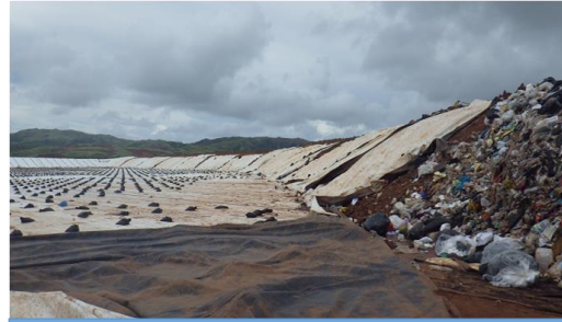
Guam's modern sanitary Layon Landfill
