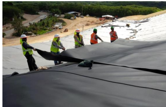
Geo-composite and geo-membrane cover pulled into place at Ordot Dump, now closed.
