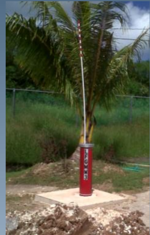
Gas monitoring well
