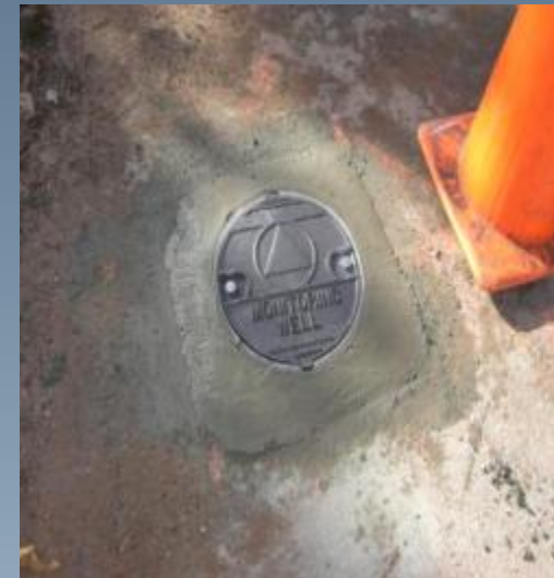
Monitoring well cap
