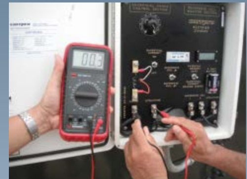
Tank cathodic protection checks
